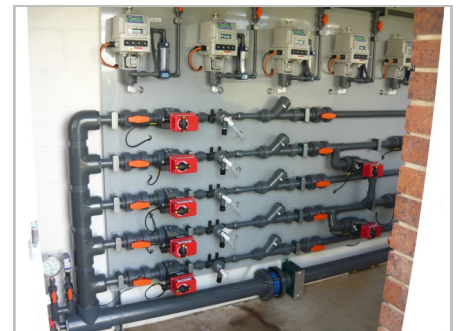
Five chlorinators & ejectors mounted on two panels with motorised actuator vales to activate which ejector they want to activate.
