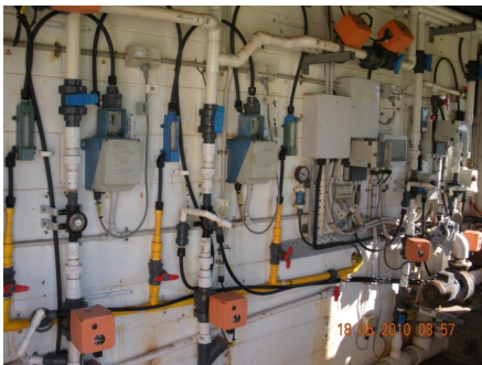
The old Fisher & Porter gas equipment had served it's time and was becoming expensive to run and also an OH&S issue. A new system had to be designed and installed.
