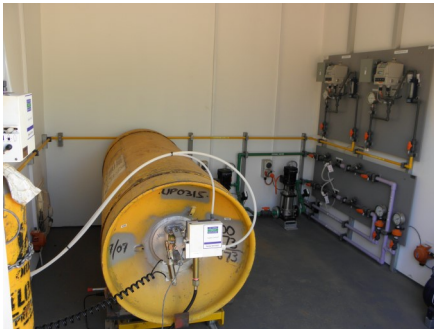
Chlorine drum mounted on a trolley and rail weigh scale system for ease of installation and storage. 1 drum last a year and they are changed over by WestWater Personnel upon service visits
