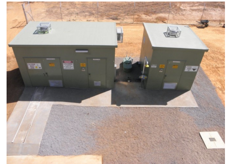
2 buildings containing chlorination, fluoridation and control systems. Pre built in Sydney and barged to site meaning installation time was only 2 weeks completely commissioned
